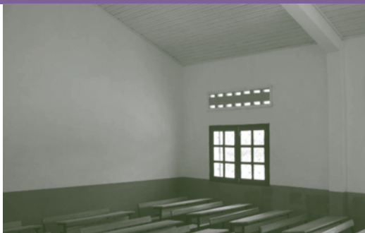
Completed classroom of Soanonanana primary school reconstructed in the commune of Vohimarina, Fianarantsoa Province
