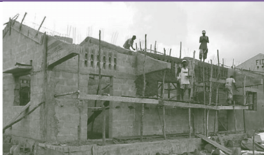
Primary school in the commune of Antombana (Antsiranana Province) with sloping roof beams made of reinforced concrete.
